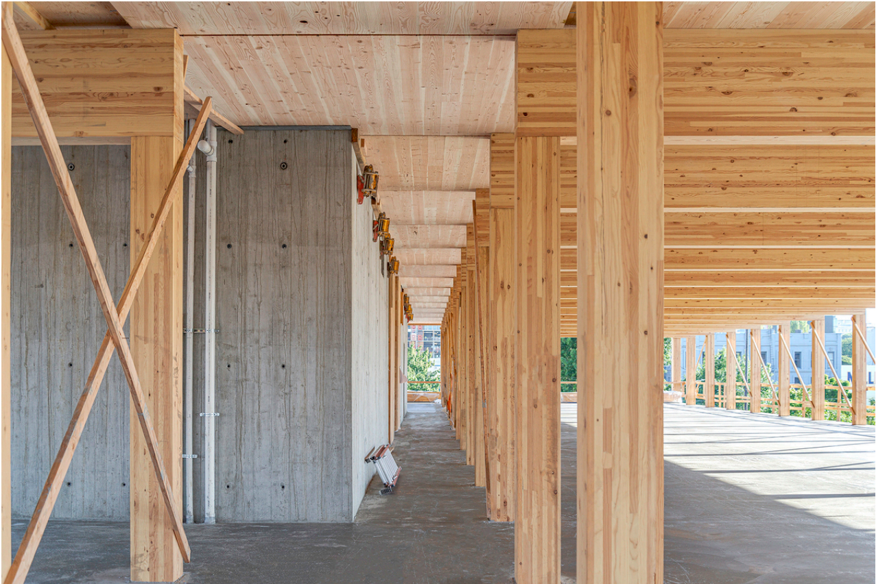
Two-way CLT is used for a beamless zone adjacent to the core at District Office in Portland, OR / Photo Hacker
