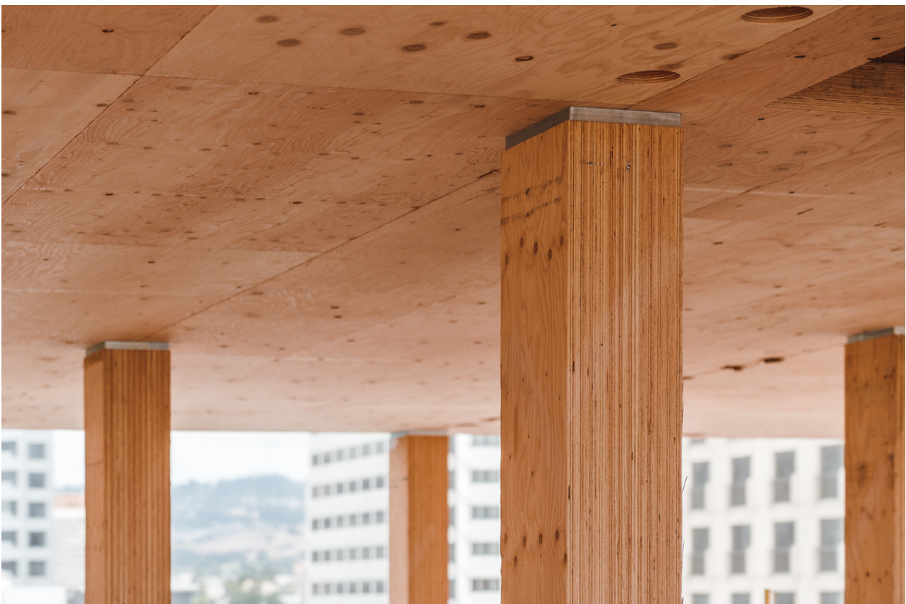
CLT panels made from SCL laminations span two ways at 1510 Webster in Oakland, CA / Photo WoodWorks
