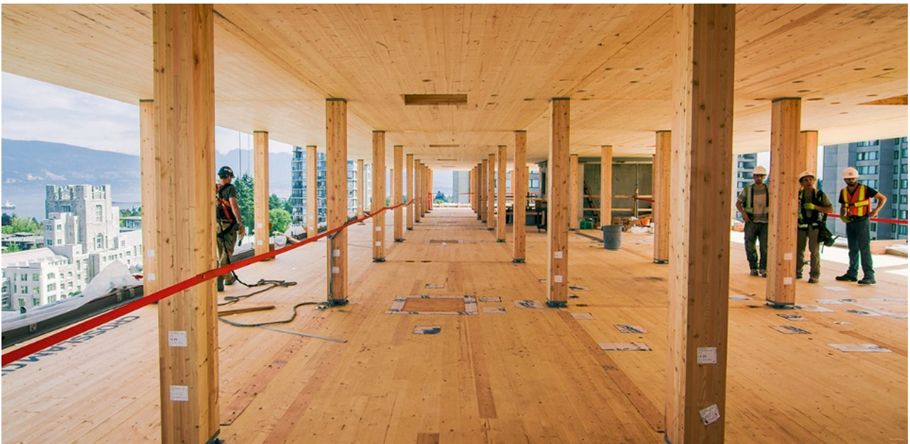
CLT panels span two ways at Brock Commons Tallwood House in Vancouver, BC / Photo Acton Ostry Architects
